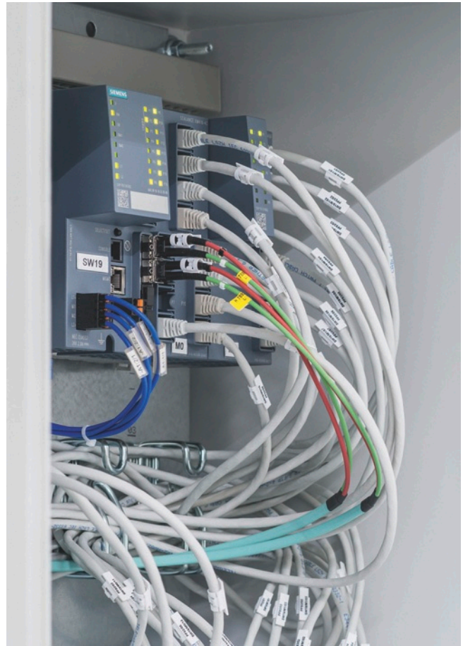
A total of 95 Scalance X switches form the interfaces of a network structure made up of multiple subnets, e.g., consisting of Scalance XM416-4C ....
