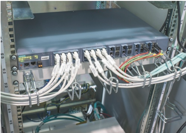
The managed switches SCALANCE XR528-6M with device network management from Siemens are connected with a 1 Gbit line.
