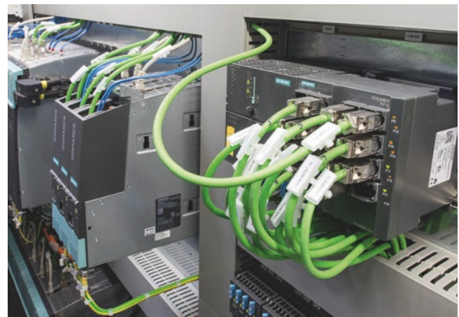
... or Scalance X216; here installed in a control cabinet.
