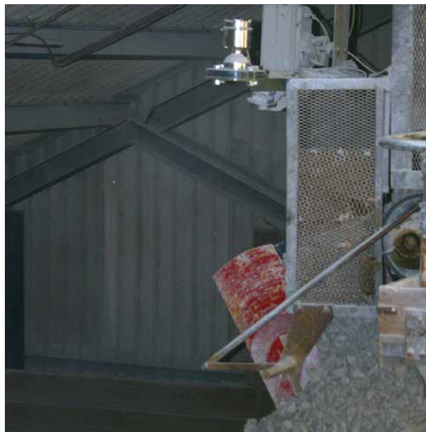
The 78 GHz SITRANS LR560 radar transmitter, mounted on this shuttle conveyor, gives precise level readings of finished clay in the storage bays.
