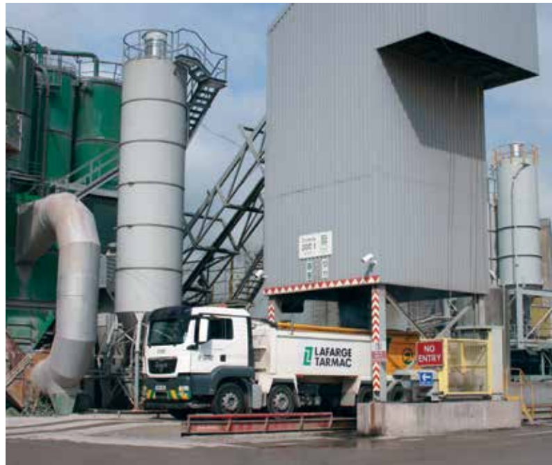
Trucks arrive daily to pick up hot asphalt from Lafarge Tarmac's finished asphalt storage silo. The SITRANS LR560 radar transmitter is installed at the top of the 10m narrow silo that houses the fibre.
