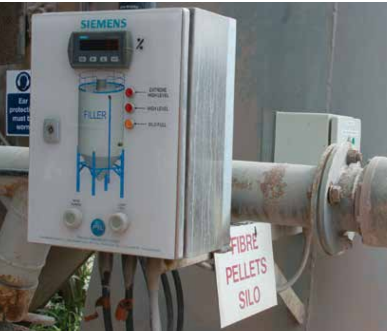
SITRANS RD200 remote display, connected to this custom-built panel, shows level percentages in the fibre pellet storage vessel.
