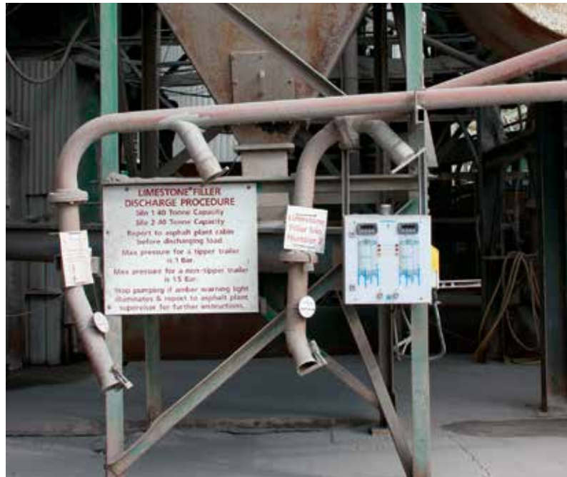
Delivery truck drivers can easily read the display panel while filling limestone dust into the two storage vessels.
