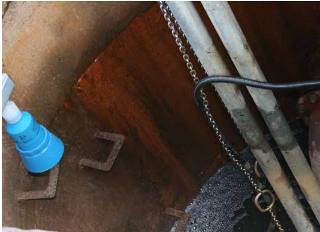
With the numerous obstructions in this wet well, including a ladder, pipes, and chains, accurate and reliable level measurement can be quite challenging.
