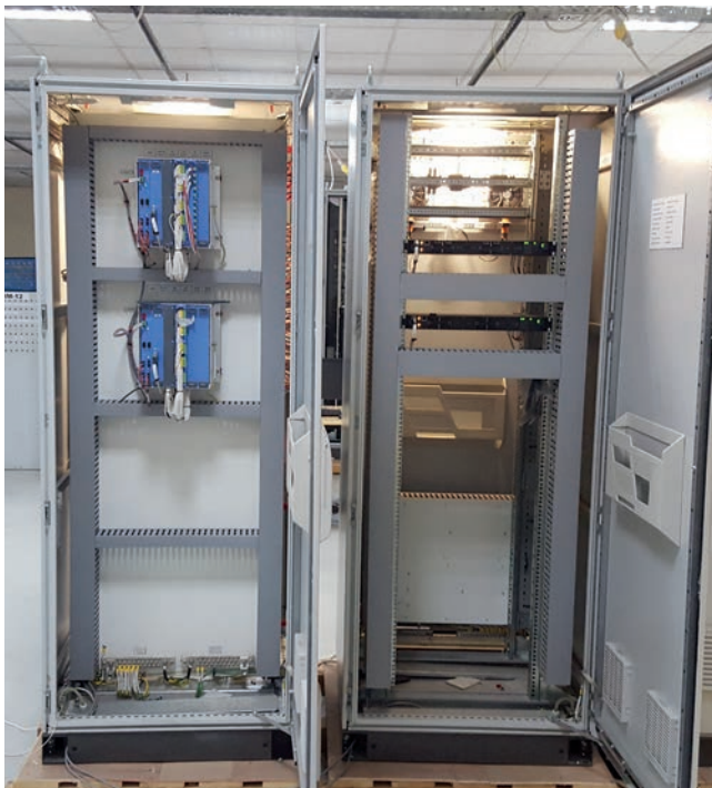
RUGGEDCOM RSG2100 switches in RTU cabinet
