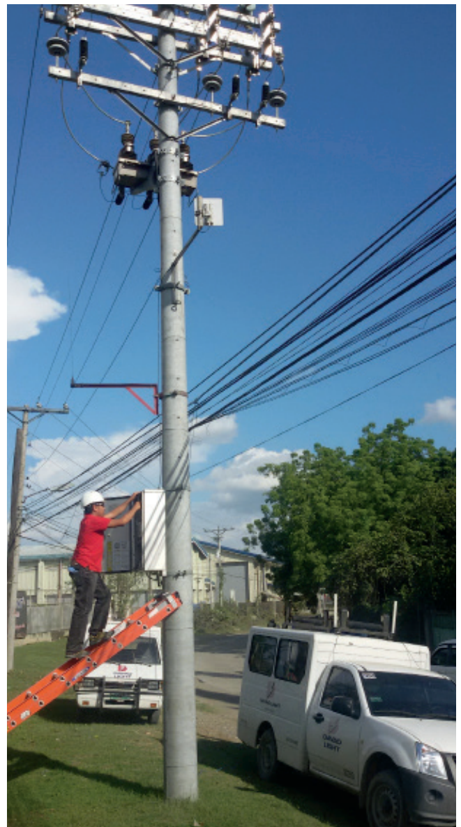
Demand response, remote disconnection
