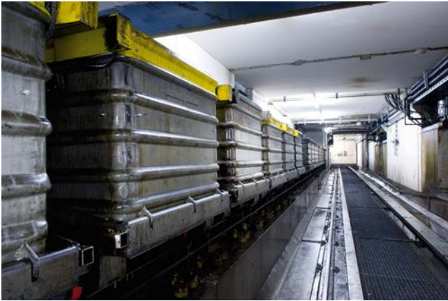
Image 2: With the new control and identification utilizing RFID technology (radio frequency identification) by Siemens, MEVACO has made the unmixed collection of stamping scrap much more flexible and future-proof
